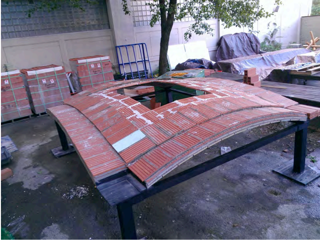
Figure10: Guastavino mockup vault under construction, showing blue insulation tile which was later covered by more tile
