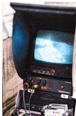
Vertical cracks in an internal cast iron roof leader were identified using the SeeSnake®
