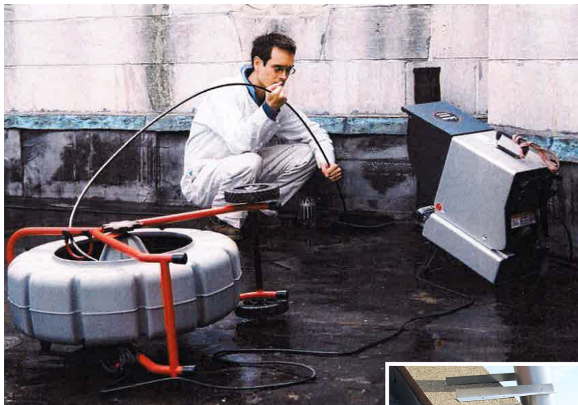
Fiber-optic investigation of a drain pipe embedded within a masonry wall at St. Thomas Church in New York City.
